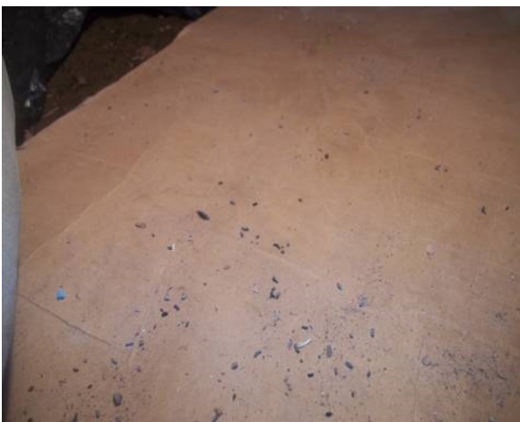
Rodent feces noted. Monitor for further presence in the future.
