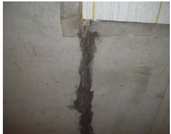
Crack / repair noted.
