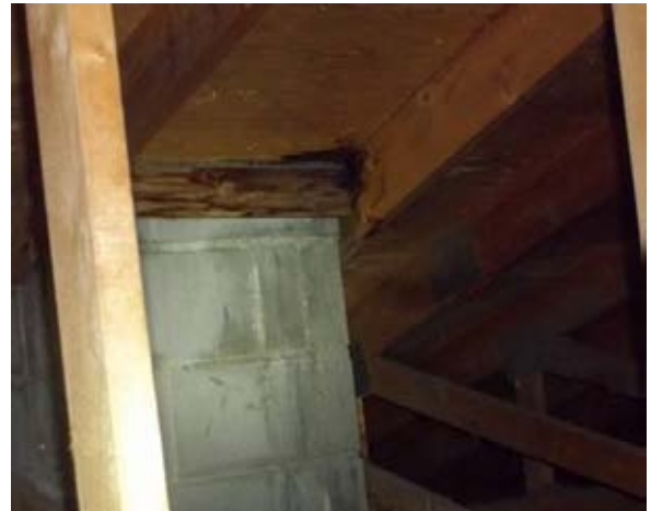
Stain noted. Dry at time of inspection.
