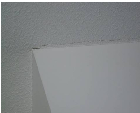
Settlement crack noted. Monitor for further movement.
